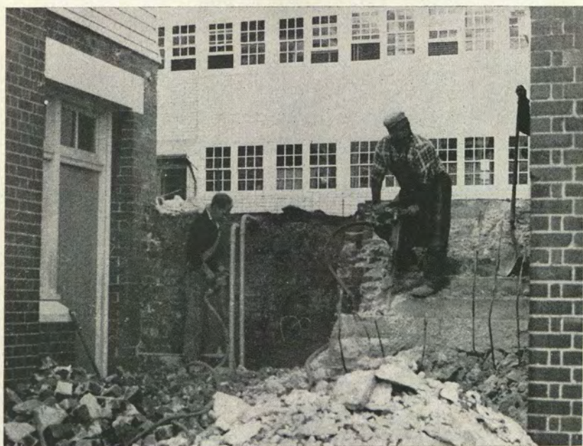
The old steps leading to the canteen area are demolished . . . with much noise!
