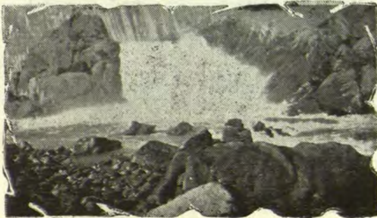
ESCAPE OF WATER THROUGH WALL OF BURRENJUCK DAM.
